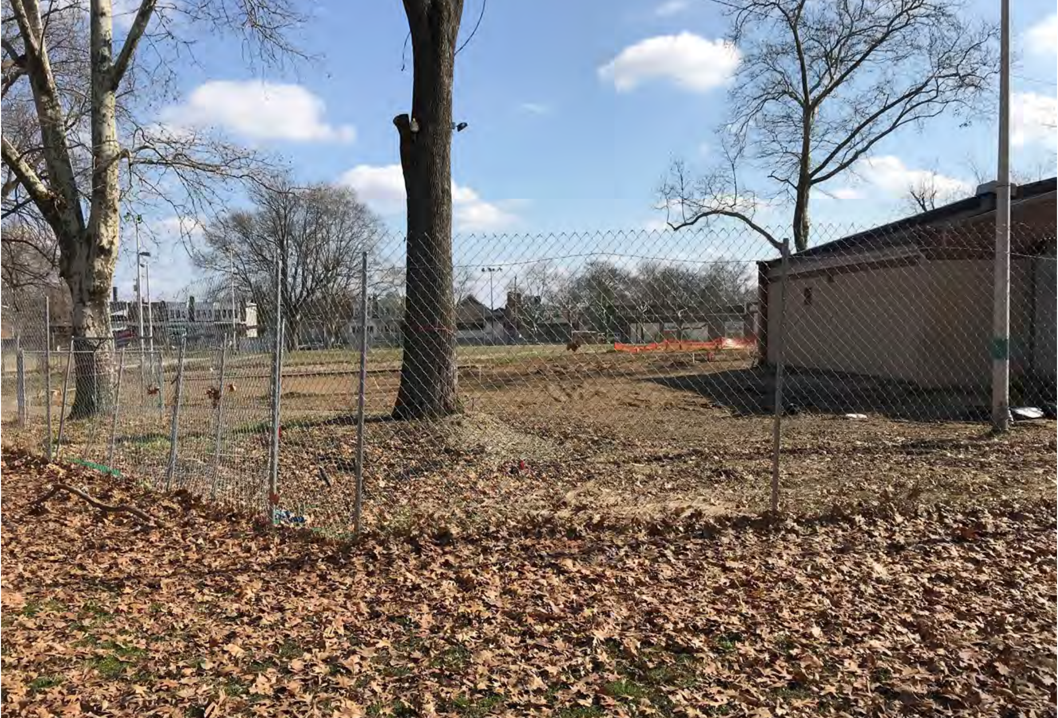
The granite base was removed from the site as part of the current renovations at the Stenton Park Rec Center between November, 2017 and February, 2018
